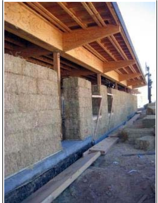
The new Santa Clarita (California) Transit Maintenance Facility features a 26,000 ft 2 (2,340 m 2 ) administration building with strawbale-infilled walls, lime-plastered on both sides. HOK is providing full architectural services.
